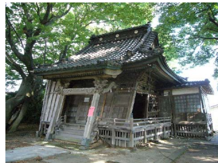
(b) damage rank D4
