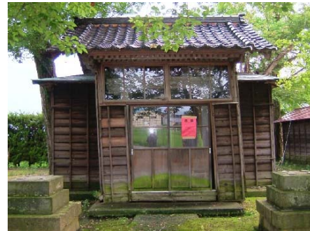
(a) damage rank D3
