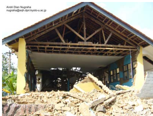
Figure 13. Damaged Yunior High School in Cigalontang-Tasikmalaya
