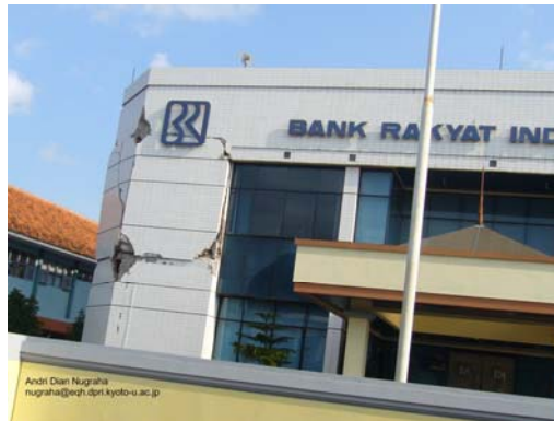
Figure 15. Damaged Bank Building in Ciamis
