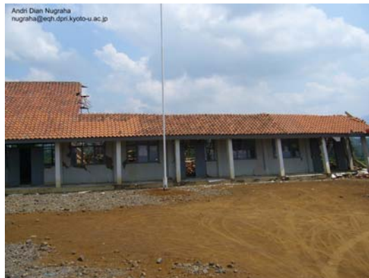
Figure 12. Damaged Senior High School in Cigalontang-Tasikmalaya
