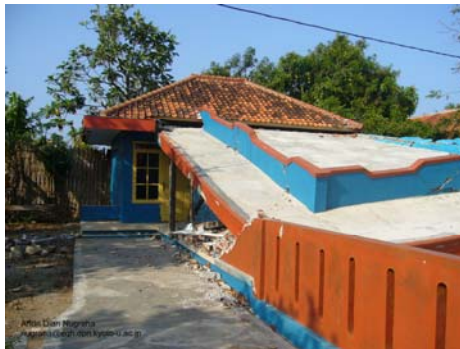
Figure 9. Damaged house in Cikelet-Garut
