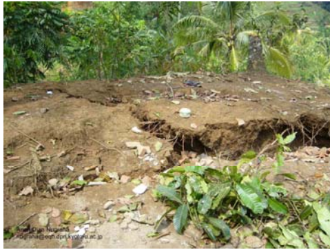
Figure 11. Ground Cracked in Cigalontang-Tasikmalaya after the earthquake
