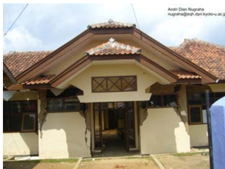
Figure 10. Damaged house in Cigalontang-Tasikmalaya
