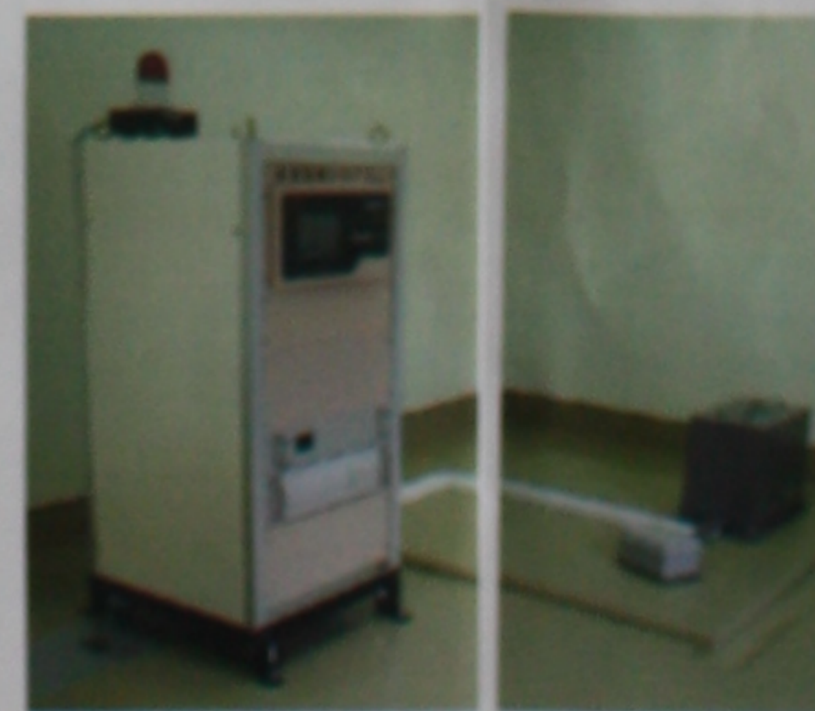
Fig.4 New EEW System (The 3rd gen)
