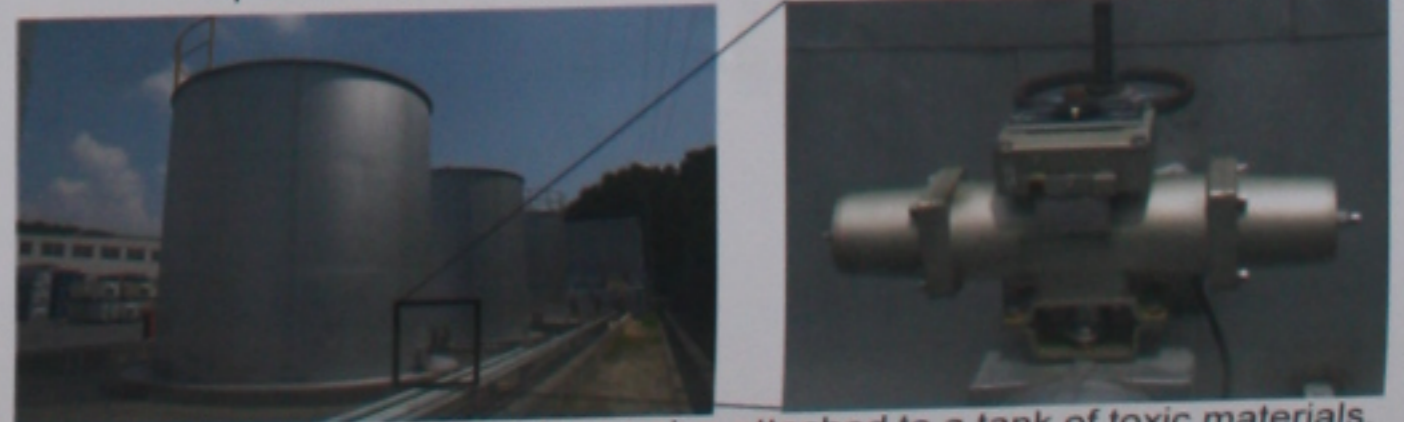
Photo 2 Example of shutdown system by a valve attached to a tank of toxic materials.
