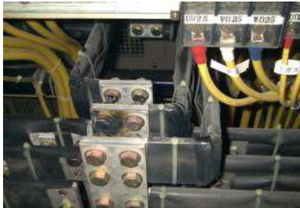
Reinforcement of copper bar
